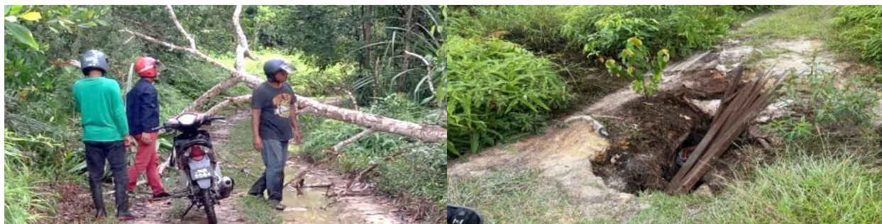
Figure 26. Fallen trees and road damage at the main access route to the planting site, FC 103 due to strong winds and strong water currents during SWM at GAFR
