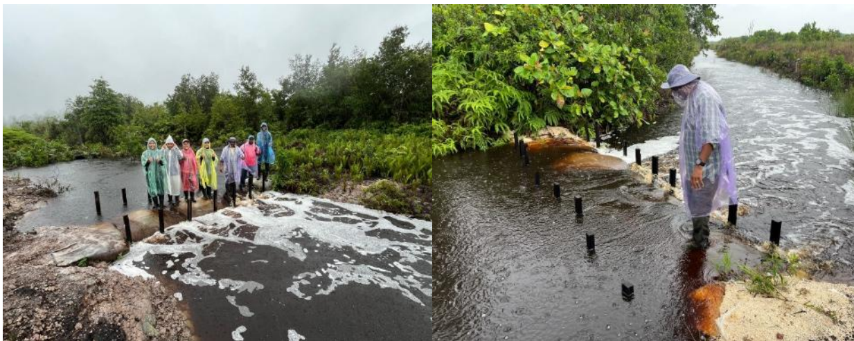
Figure 12. Monitoring and check on the canal blocks built at Parit Sembilan, Air Papan, Mersing, Johor, conducted during the monsoon season in December 2025 to ensure the stability, strength and functionality of the structure.
